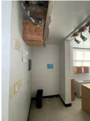
Figure 3.6.3 Damage and paint peeling from Intake Area 12
