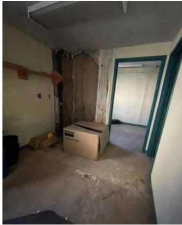
Figure 3.6.6 Water damage located on the walls and floors of Office 12
